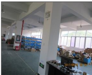
Photo of fire safety equipment Evacuation indicating signs and emergency lights at passageway 1.JPG
