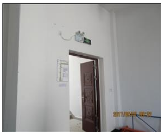
Photo of fire safety equipment Emergency exits.JPG
