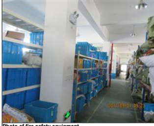
Photo of fire safety equipment Evacuation indicating signs and emergency lights at passageway 2.JPG
