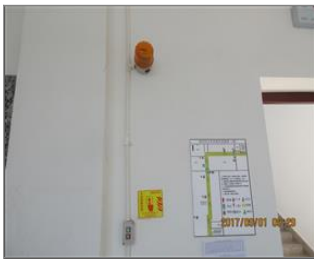
Photo of fire safety equipment Fire alarms.JPG
