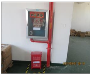
Photo of fire safety equipment Fire extinguishers and fire hydrants.JPG
