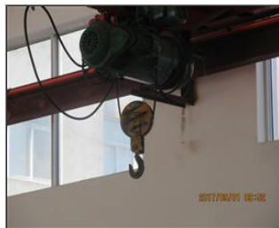
Photo of non-conformity No safety catch.JPG
