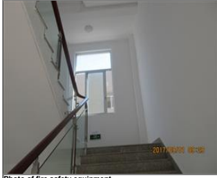
Photo of fire safety equipment Evacuation indicating signs and emergency lights at stairs.JPG
